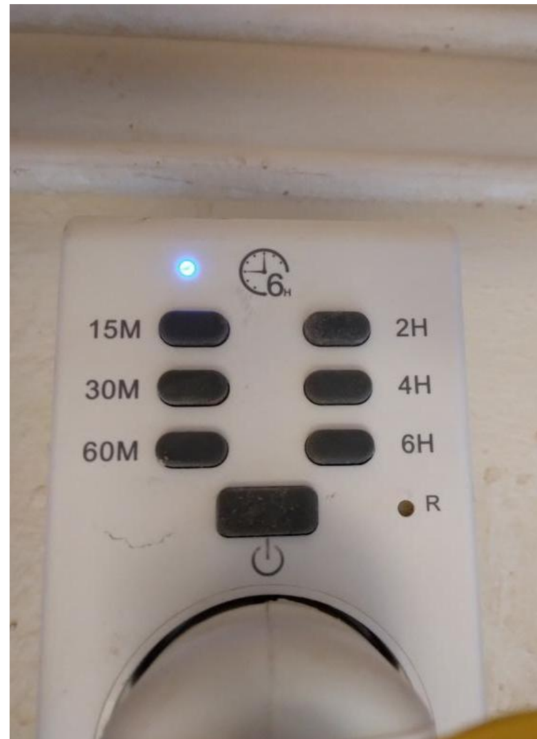
Figure 7: The ventilation timer is on
