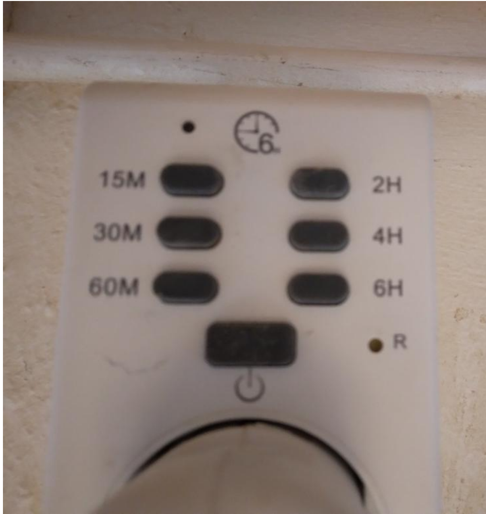
Figure 6: The button on the ventilation timer
