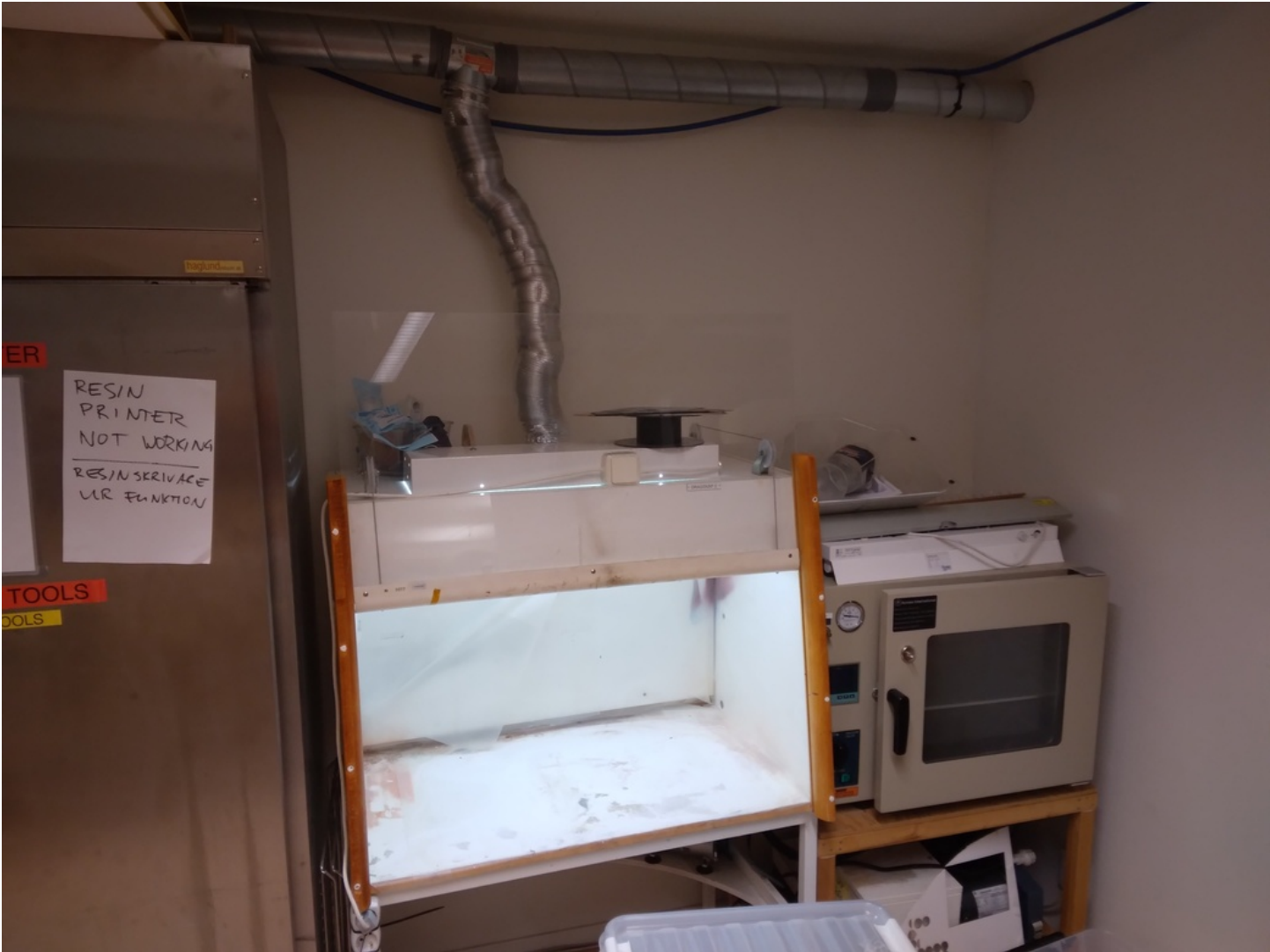
Figure 8: The fume hood
